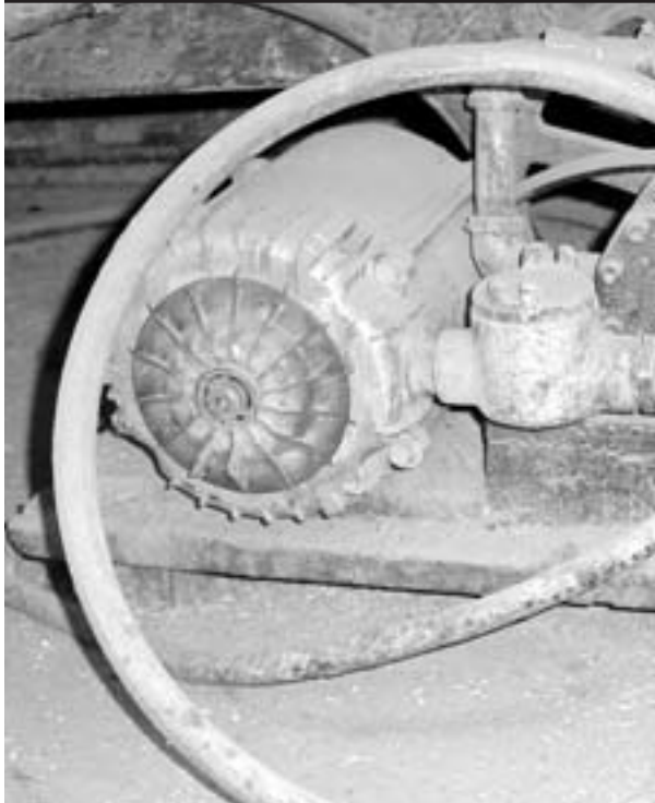
Circulating tank pump
