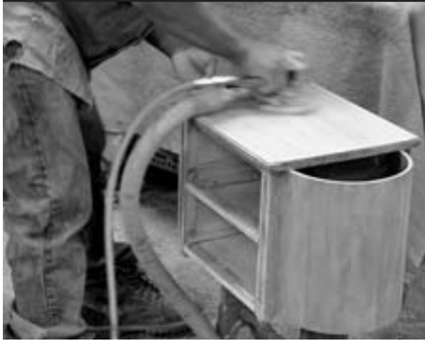
Strip excess coats of paint with sandpaper before applying the paint stripper.
